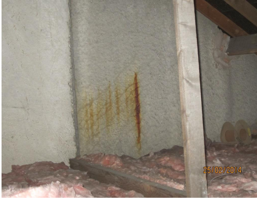
Rusting Reinforcement to party wall in roof
