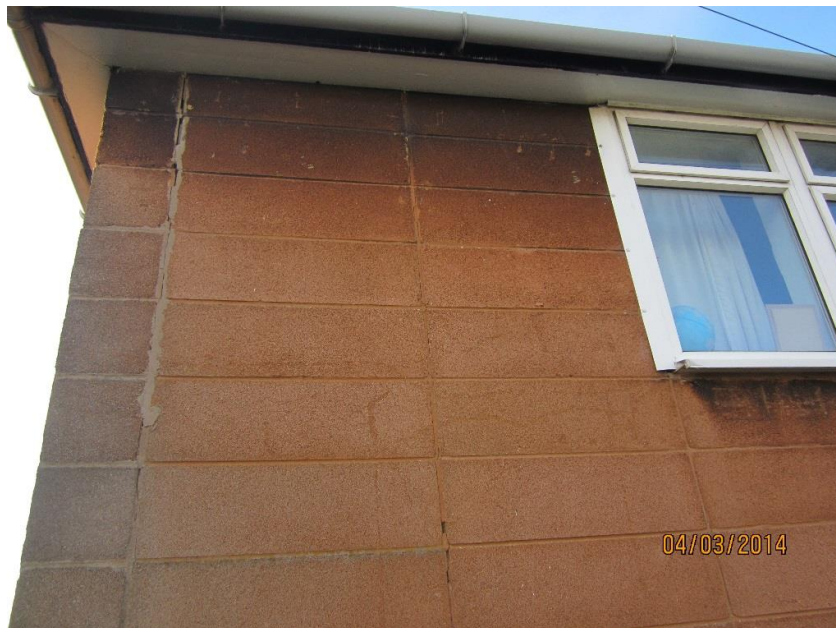
Cracked & Open Joints
