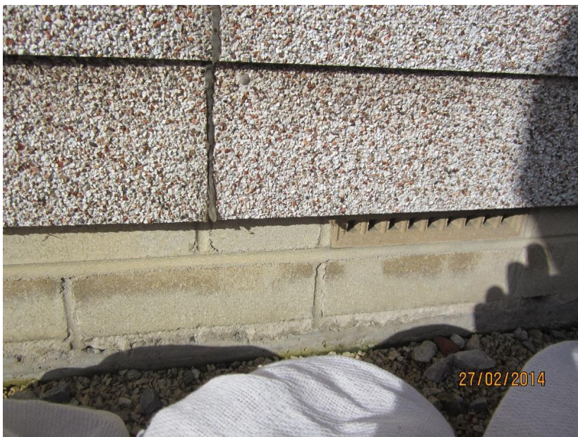
Existing Cladding Obstructing Ventilation
