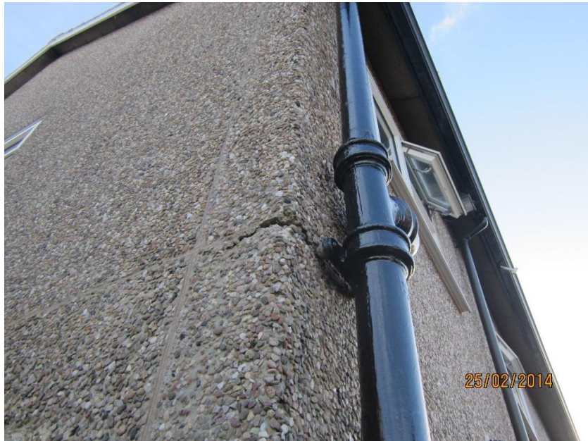
Cracked & Spalled Concrete
